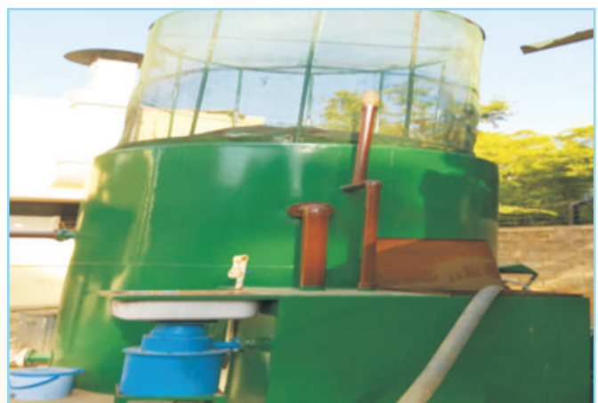
Kitchen Waste Biogas Plant at UG Girls Hostel, GKVK
