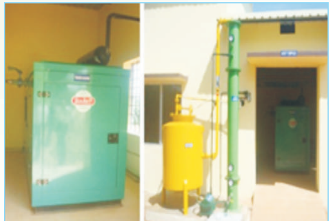
Biogas Power Generation Unit
