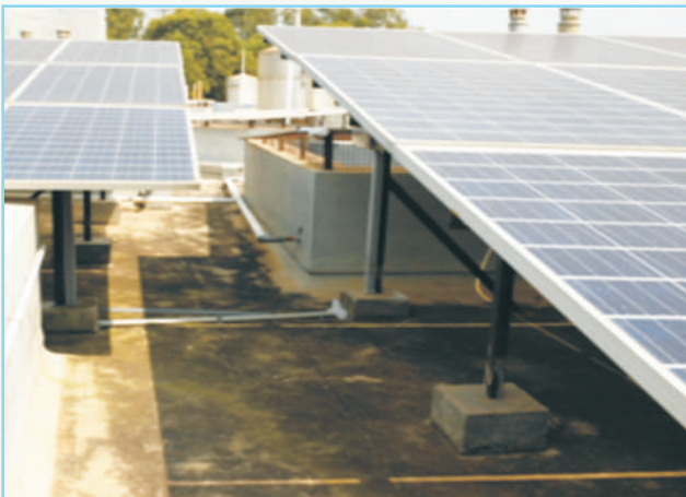
Roof Top Solar Power Plant at Hostel
