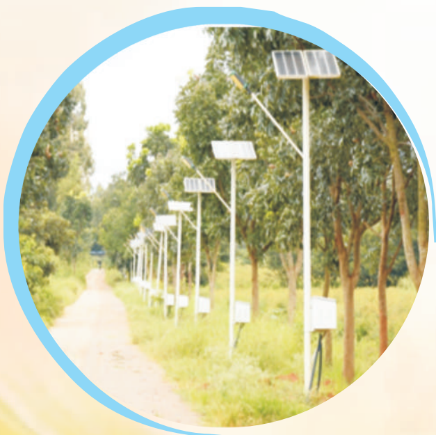
Solar Street Lights at GKVK Campus
