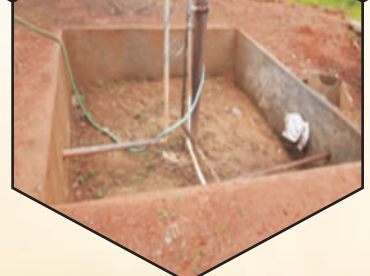
Borewell Recharge System
